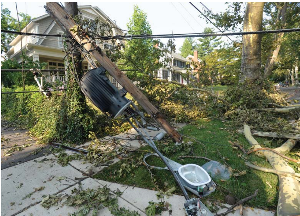
In 2013 the Commission was studying the question of whether Pepco should underground cables in neighborhoods that are historically prone to outages caused by storms.
